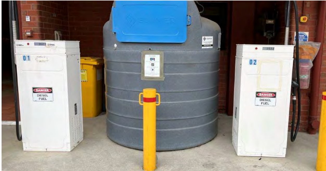
Photo 9 Fuel bowsers above underground storage tanks, located to the north of the 'No. 2 Engine Room'
