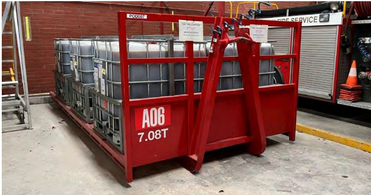
Photo 1 'Foam pod', ready for loading to rear of MFS vehicle, stored in the 'No 2. Engine Room', central-southern portion of site
