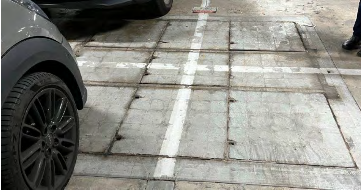
Photo 7 Stormwater collection pit, central within basement carpark, Main Building
