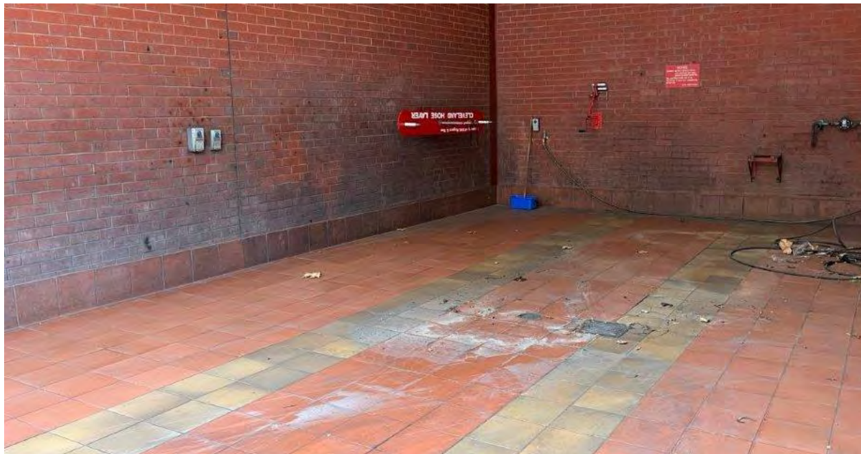
Photo 10 Interior view of the wash down bay, eastern end of the 'No. 2 Engine Room', looking south-east
