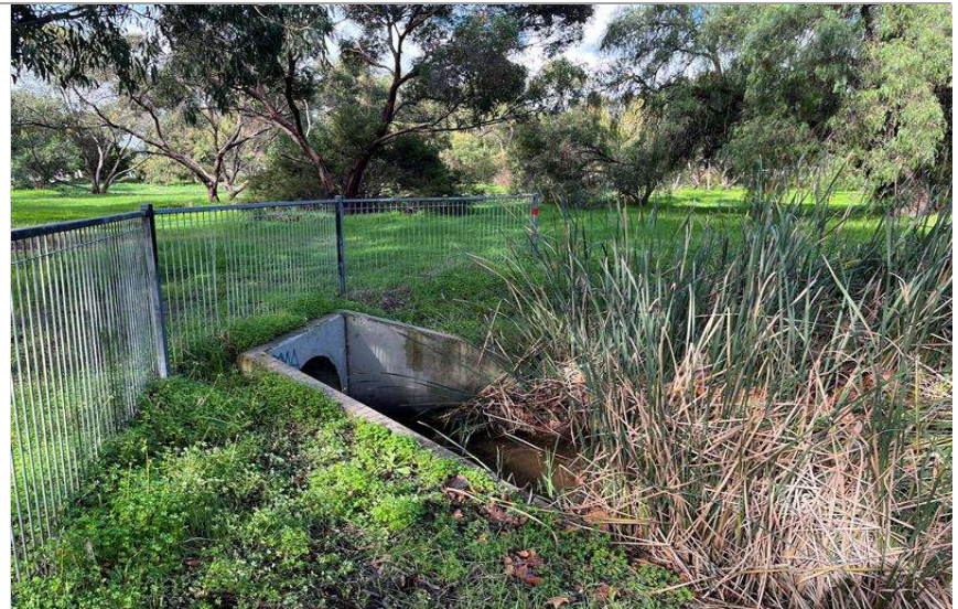
Photo 4 Sampling location PL_SW01
