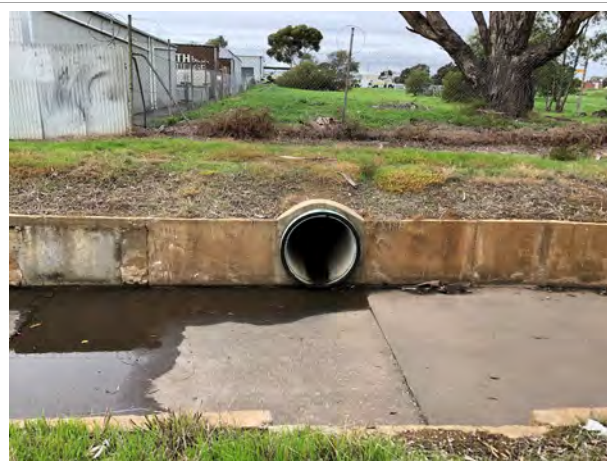
Photo 6 Open stormwater drain at the north-western site corner, facing east
